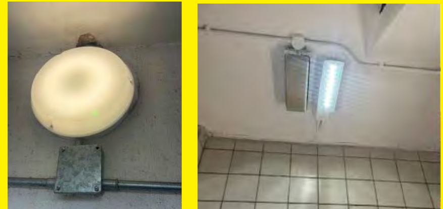
Emergency lights at 23-34 Primrose Hill Court.
