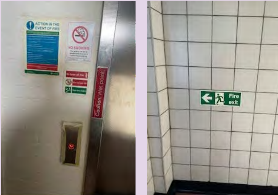
Fire Action Notices and Fire Exit Signs at 23-34 Primrose Hill Court.
