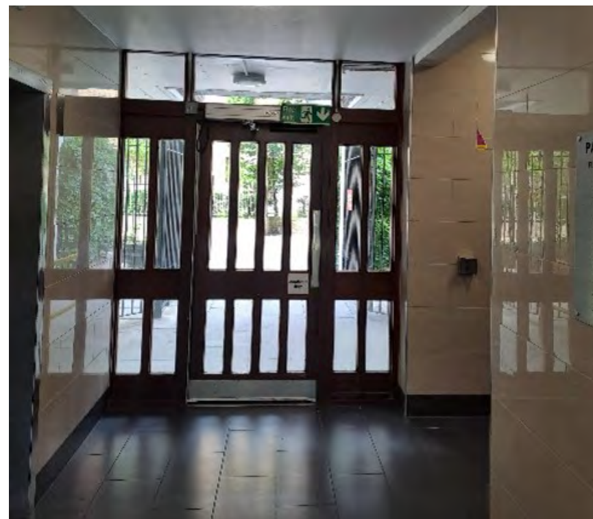
Communal Fire Door at Palgrave House.
